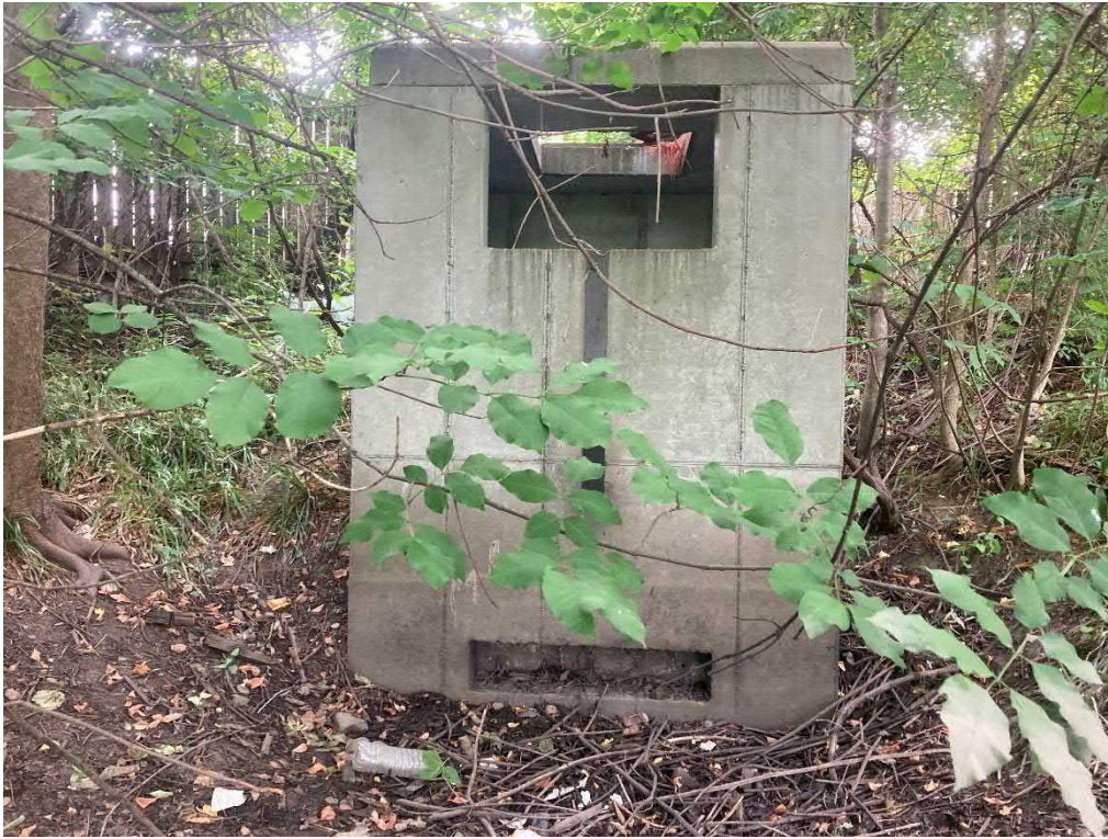
Detention Basin PS-01 (stormwater inlet) facing northeast on July 8, 2021.
